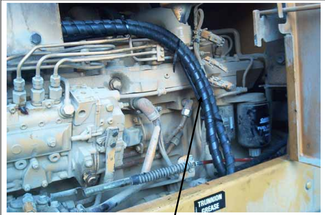
Hoses from compressor going to evaporator and condenser.
