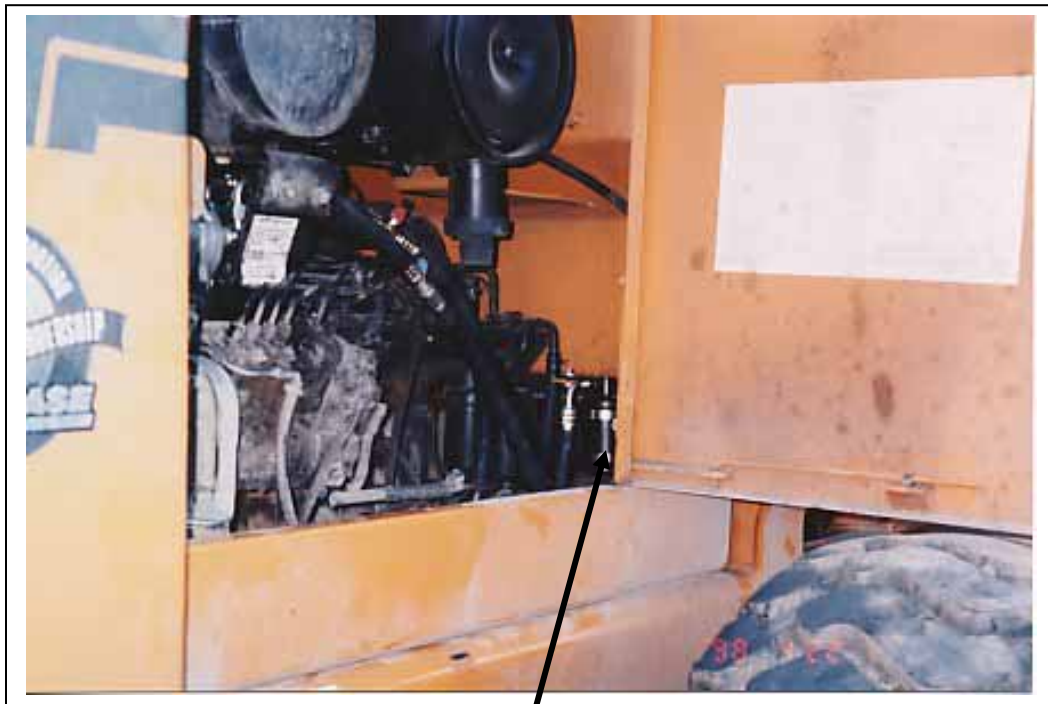
Drier mounted on front wall of engine compartment.
