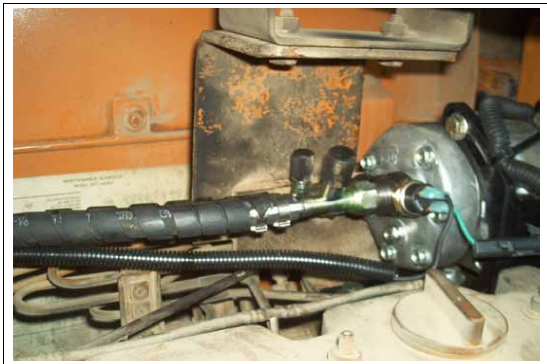
Back view of compressor
